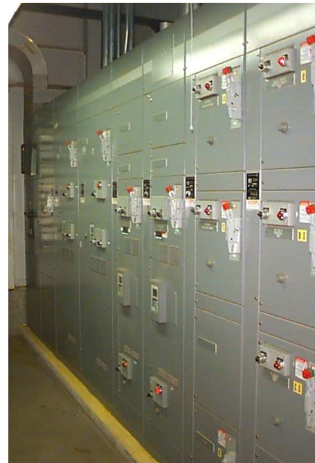
Figure 4: Variable Frequency Drives
