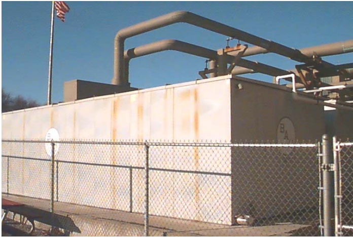
Figure 3: Building 12 Ice Storage System
