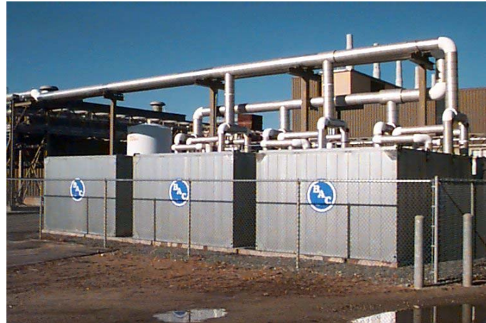
Figure 1: Building 11 Ice Storage System
