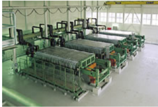
AGC chloralkali plant
