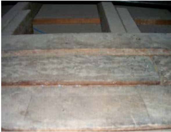
Lead dust in ceiling space
