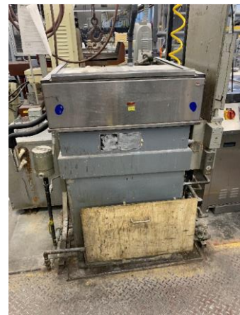
Old vapor degreaser that used TCE
