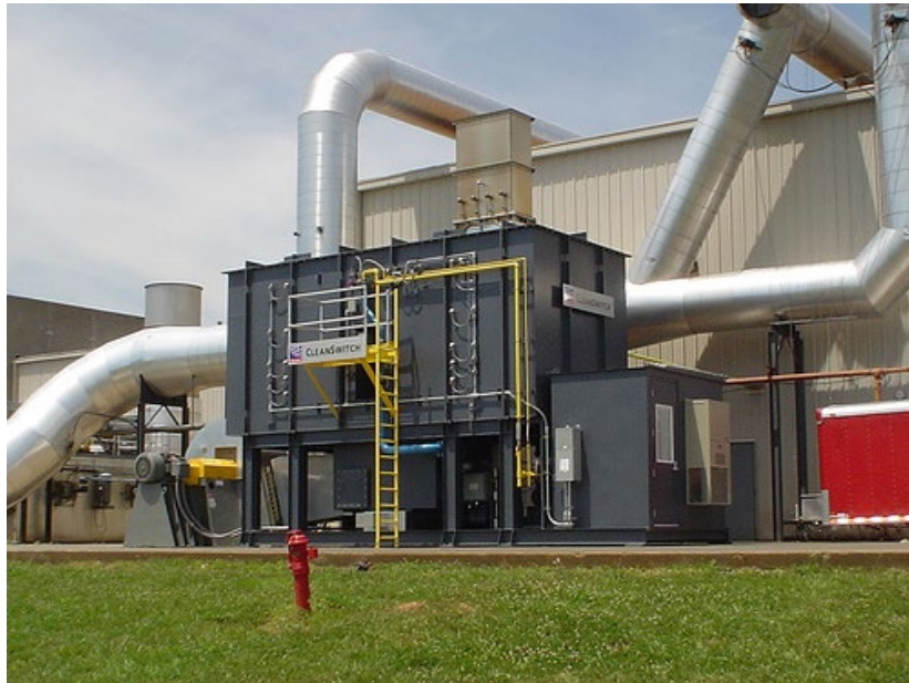
Heat recovery oxidizer used to burn VOCs
