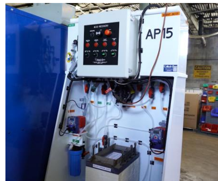
The Mech-Chem AP-15 system used by River Street to filter sulfuric acid
