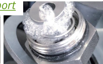
Figure 1: Polymerized refrigerant in connecting piece
